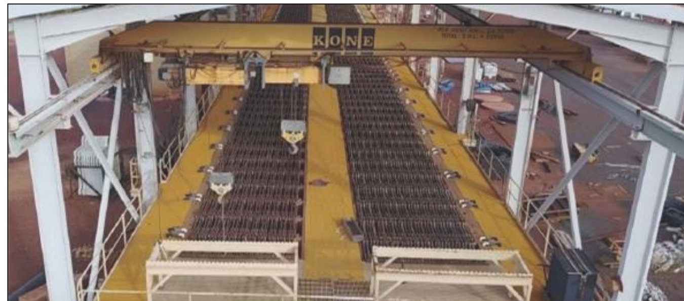
Partial refurbishment of Electrowinning Circuit to operate at 6,000 tpa, well below peak production of 25,000 tpa
